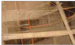
Stainless steel screens after less than six months.
