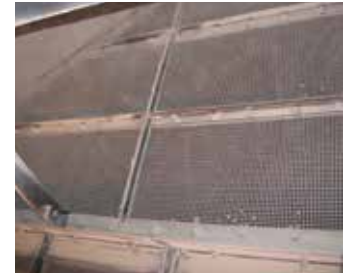
Kennametal screens after nine months.
