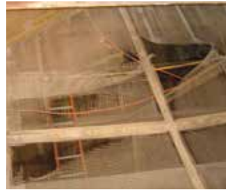
Stainless steel screens after less than six months performance.
