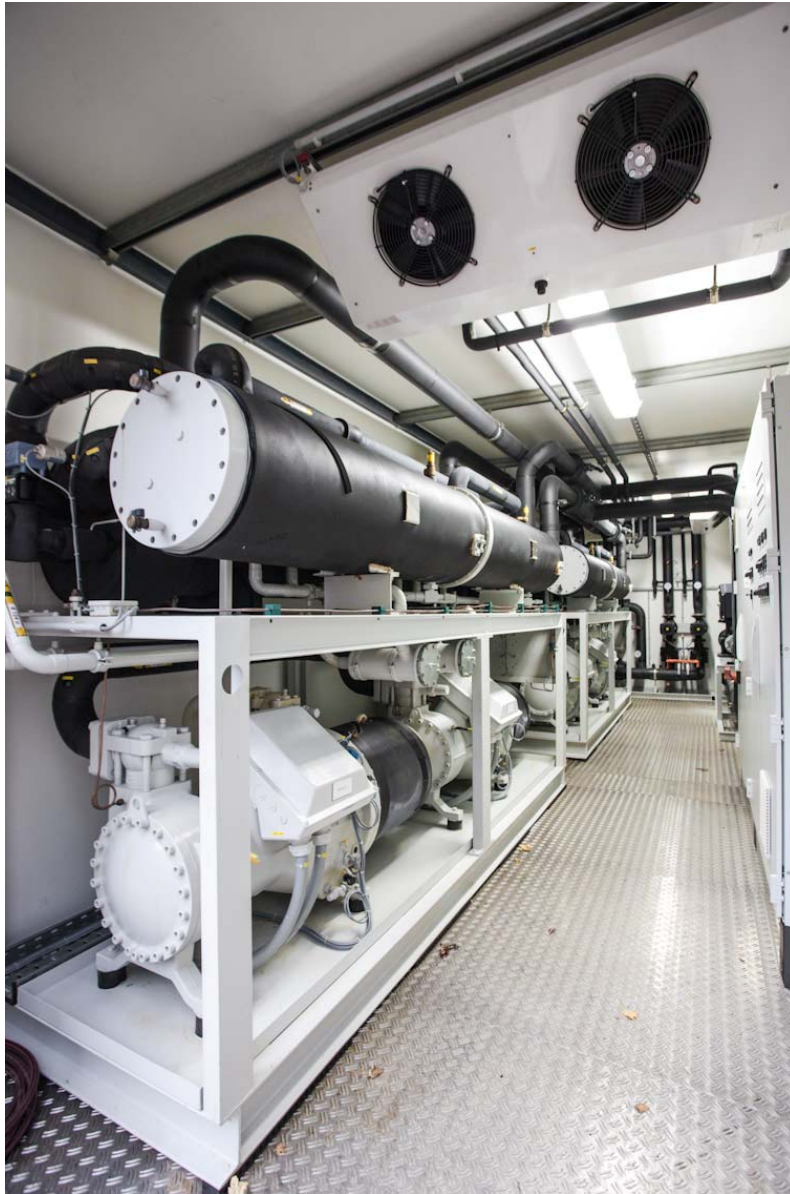
Figure 3: Industrial heat pumps installed alongside a G3516H gas generator set in a district energy plant in Reutlingen, Germany.
