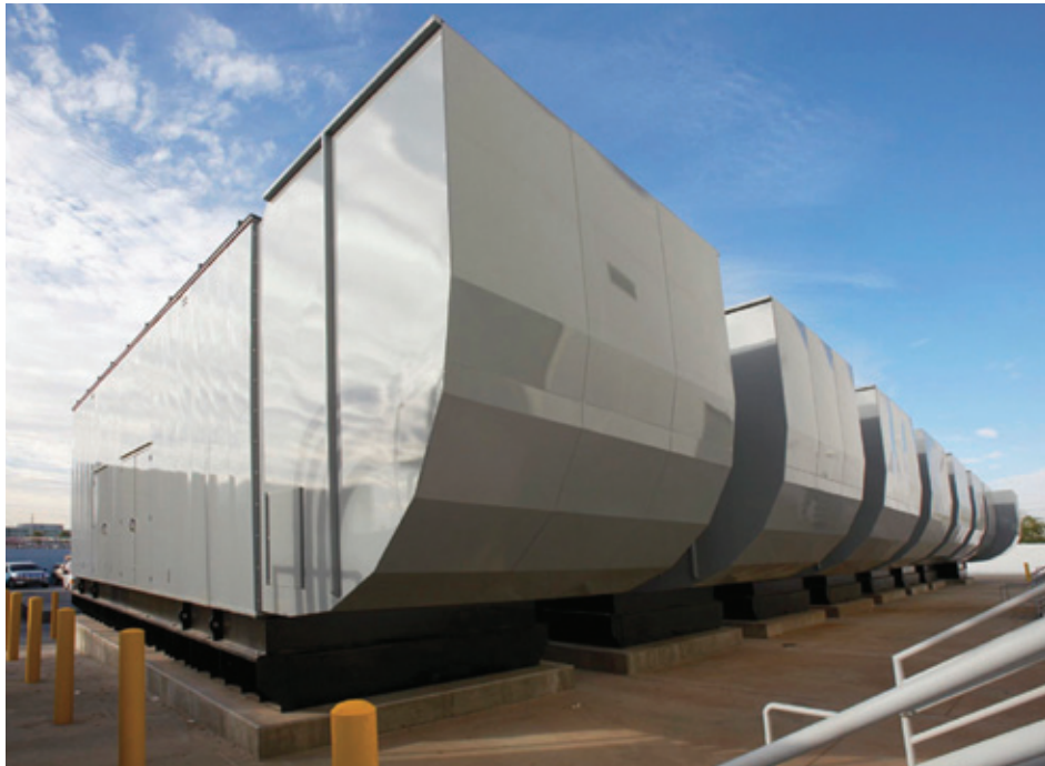
IO DATA CENTERS – PHOENIX, ARIZONA, USA
