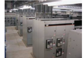
UPS Output Gear
