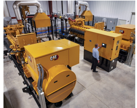
The gensets are operated remotely from the Utah Municipal Power Association headquarters 35 miles away in Spanish Fork. Operators there see the same information that appears on the switchgear HMI screen at the Nephi plant.
