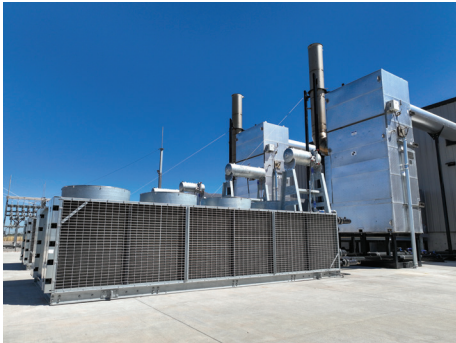
The Utah Municipal Power Association recognized that peak shaving would save money for their residents, and that without additional power they would risk blackouts. They worked with Cat® dealer Wheeler Power Systems to build a 4,732 sq. ft. power plant.
