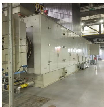
16.5 MW Turbine Generator Set Source: University of Michigan
