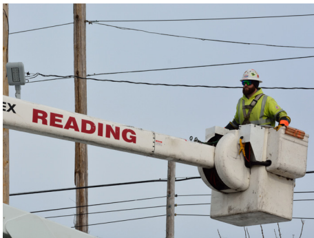
Reading Municipal Light Department has the largest electrical load among the 41 municipal light departments in Massachusetts, serving nearly 80,000 residents and more than 4,000 commercial and industrial customers.
