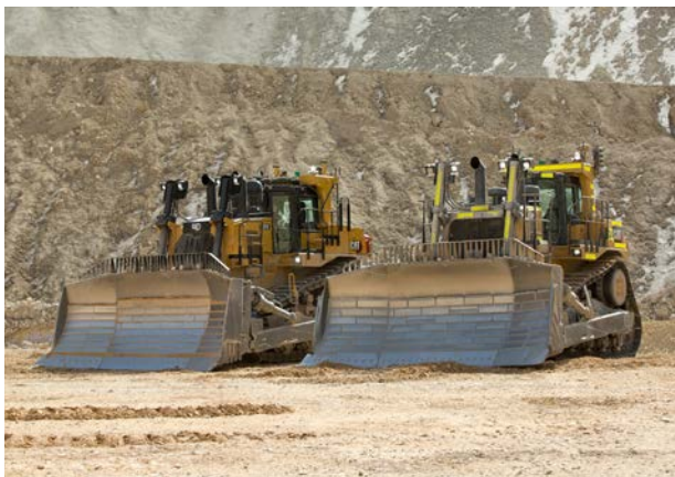
Figure 2. Caterpillar compared the performance of the new D10 (left) against the D10T2 (right) at an opencast mine, over a three-day test period.
