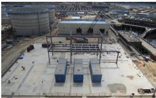
Three – 4,667 kW Solar Mercury 50 Gensets SOURCE: DC WATER
