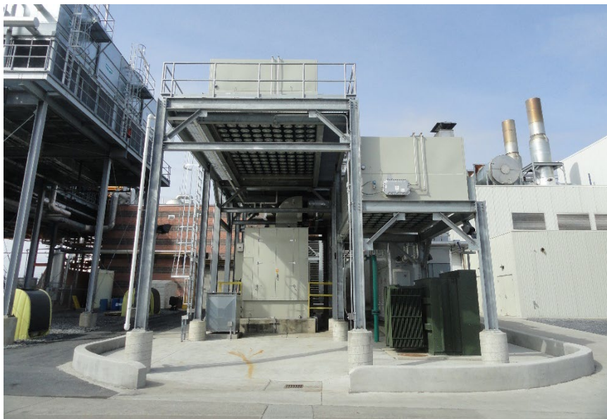
14.5 MW Packaged CHP System
