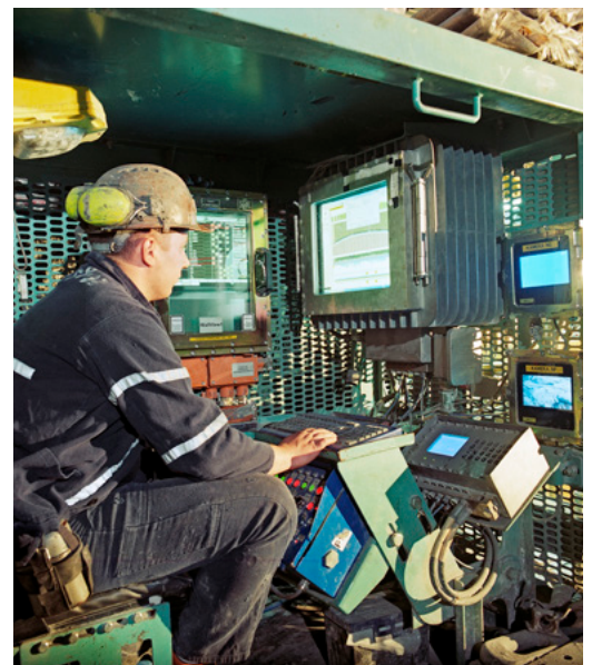
Underground control station
