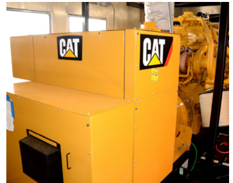
The Cat® G3512 generators were chosen because natural gas is more readily available in an emergency. The gas gensets also comply with the required standby power specifications.
