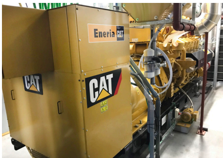
Eneria Belgium designed and installed a combined heat and power (CHP) system that features the high-efficiency Cat® G3512H gas generator set.
