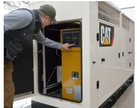
The district opted to install a Cat® DG150-2 natural gas-fueled generator set for reliable backup power.
