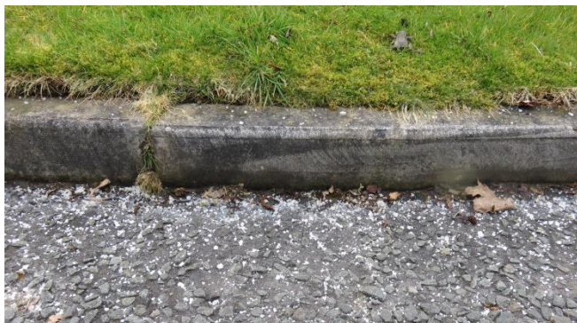
Large collection of salt collected along the kerb during spreading. Toads trapped along the kerbs succumbed quickly to the very high concentration of salt.
