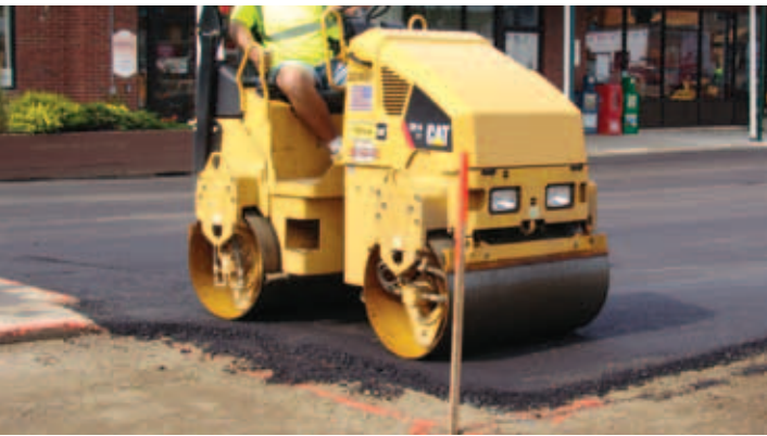
Utility-size compactors make it easier to compact around obstacles without tearing the fresh asphalt.
