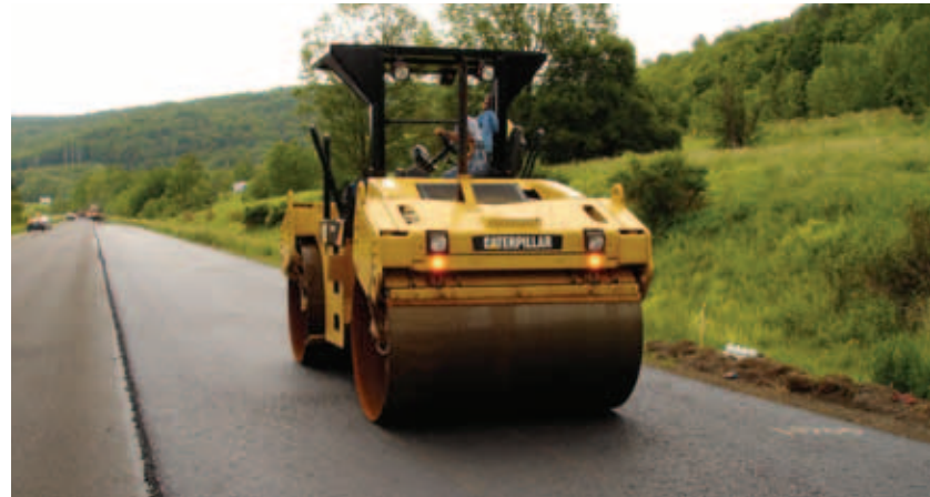
Vibratory rollers used in the intermediate phase are set to low amplitude.
