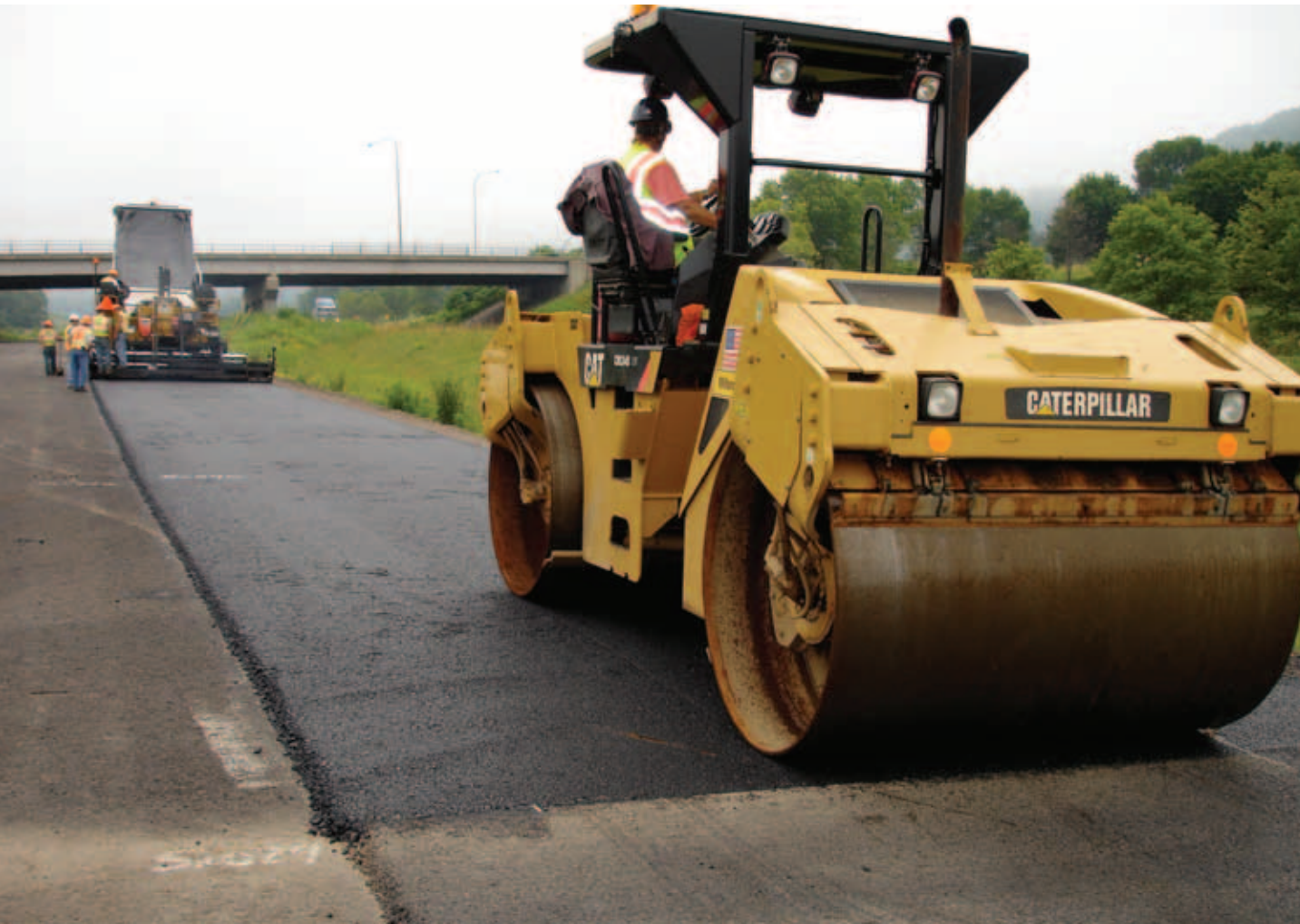
Initial compactor starting first pattern and cleaning up stop marks left during joint compaction pattern.
