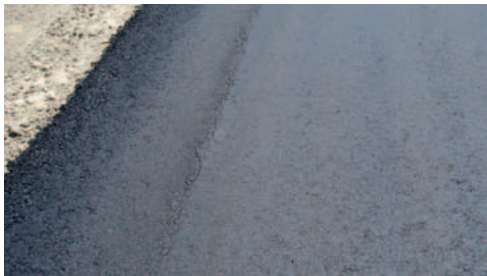
Crack in the mat along drum edge set back from the unconfined edge.
