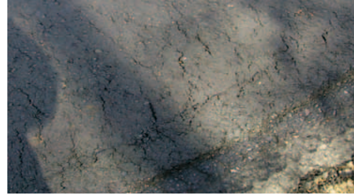
The outer edge of the drum stretched and distorted the fresh asphalt.
