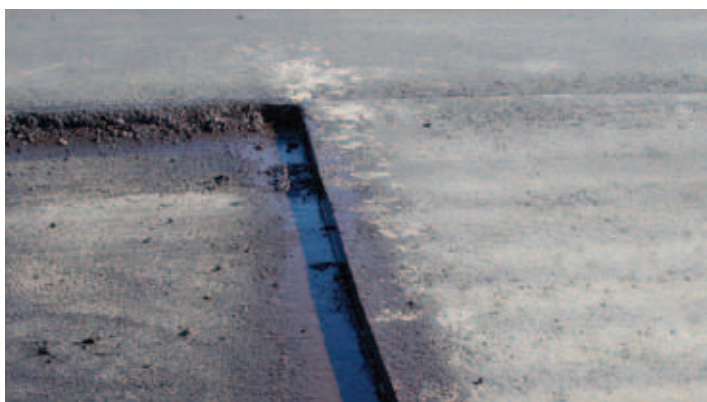
Example of a good saw-cut joint that has been tacked prior to the start of paving.
