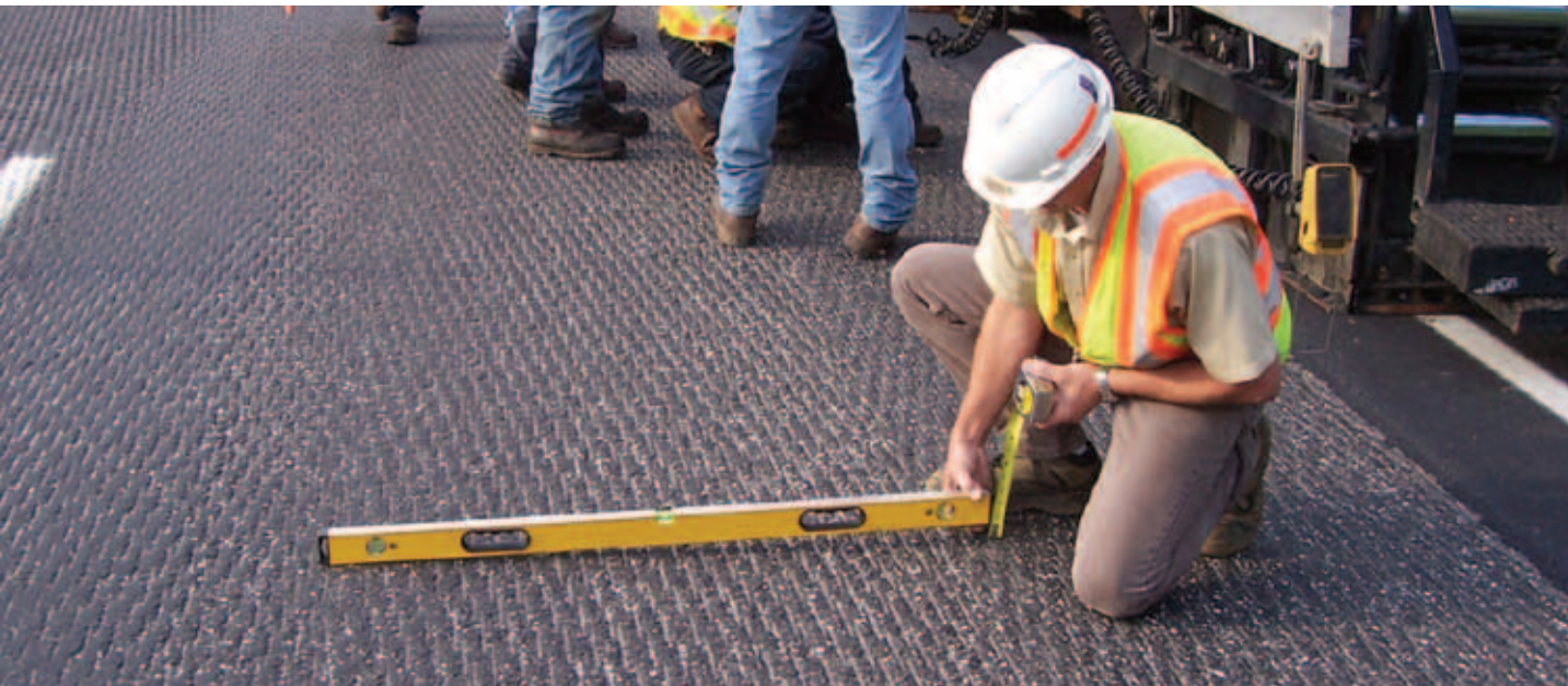
Mat thickness can be variable when slope control is used by the paving crew.
