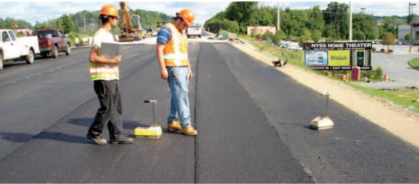
One sign that the compactor is working in a tender zone is a rolled over and cracked drum edge cut mark.
