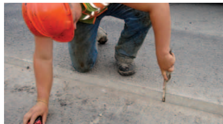
Checking the thickness of the starting joint helps the crew select the correct starter board thickness.
