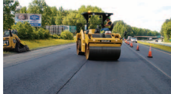
There are no drum stop marks in the fresh mat when the compactor is able to roll onto a cold, compacted mat.
