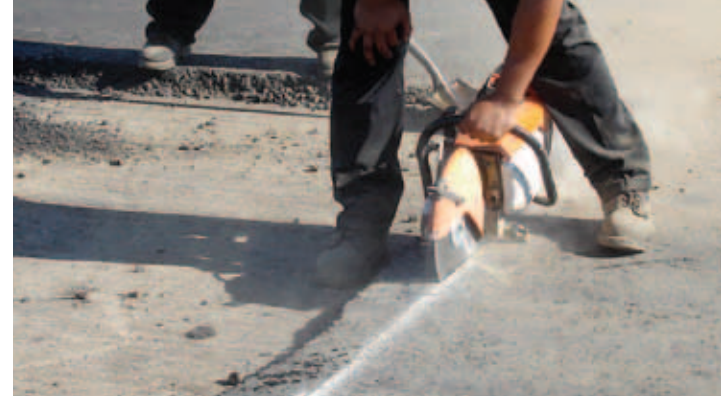
Cutting or milling a straight vertical face is a requirement for a transverse joint.
