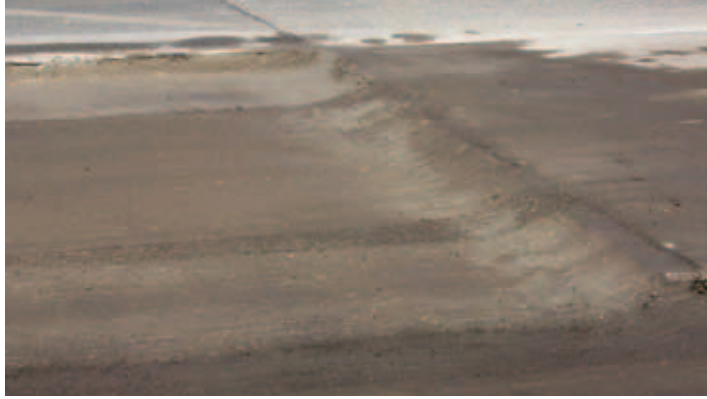
Example of a poor starting reference. Rounded face with deep plunge cut will hinder compaction.
