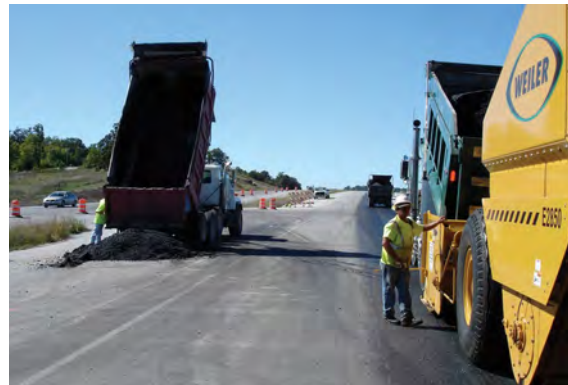
On this project, drivers use the emergency lane as a designated area for vehicle cleaning. Material will be salvaged at the end of the shift.
