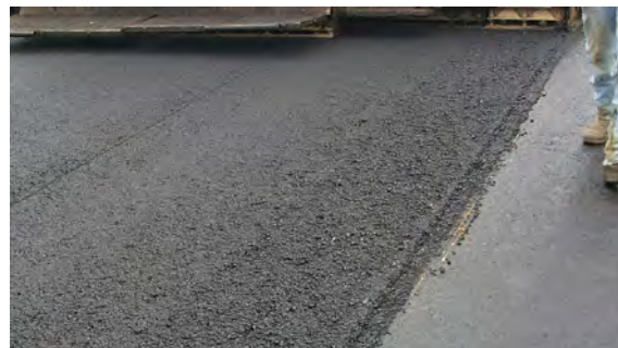
Paving with automatic slope control to correct the transverse profile created a thin layer of material on the right edge, resulting in incorrect yields.
