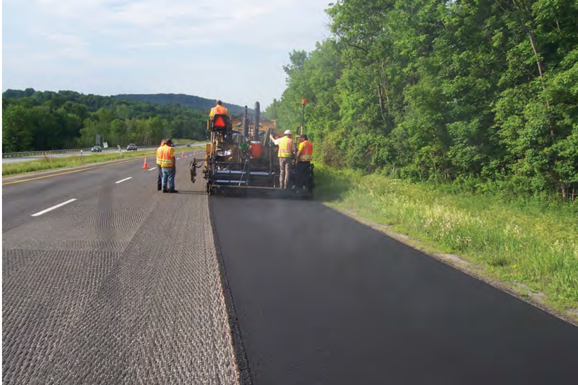
Paving the emergency lane first provides a better reference for the grade control system when paving the adjacent driving lane.
