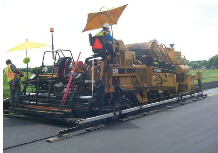
Cat 9-meter (30') multi-articulated outboard leveler averaging adjacent layer, while matching the longitudinal joint.
