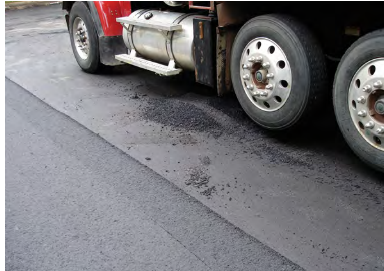
Spills in front of the paver can cause high spots in the grade.
