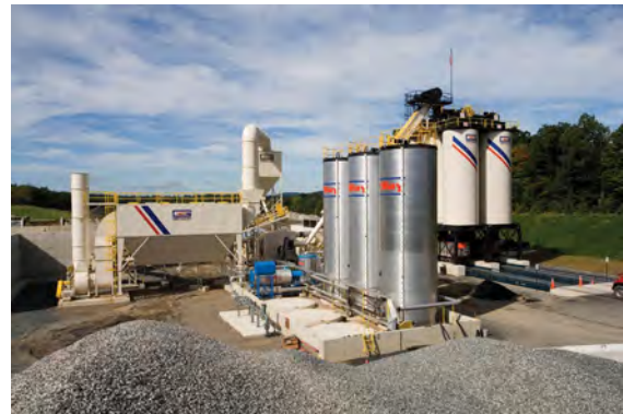
Storage tanks for asphalt cement.
