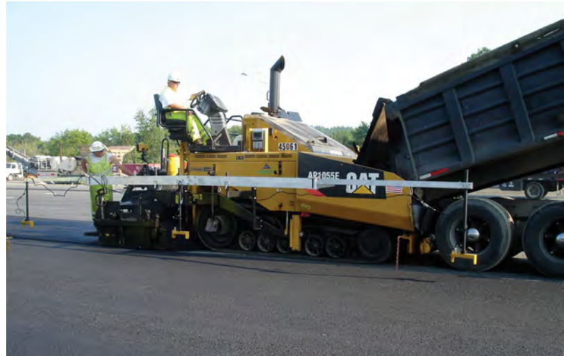
Cat non-contact averaging ski installed to reference grade outside the paving width.
