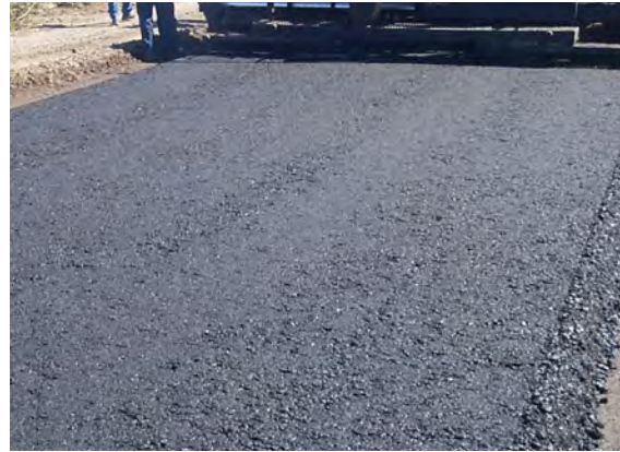
Continuous segregation stripes often relate to high auger speed.
