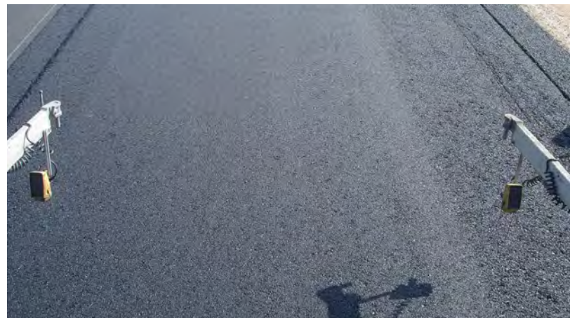
Texture stripes in the surface of the bituminous layer are usually caused by variations in the angle of attack across the width of the screed.
