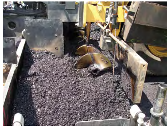
A well-trained crew has set up the feeder system to maintain the correct head of material.
