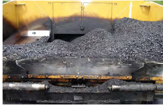
Severe segregation in the hopper caused by cycling the hopper wings when the level was too low.
