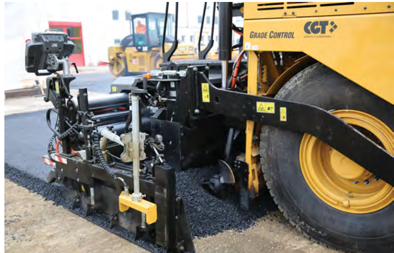
Grade sensor position just ahead of the auger chamber helps create fast screed reaction.
