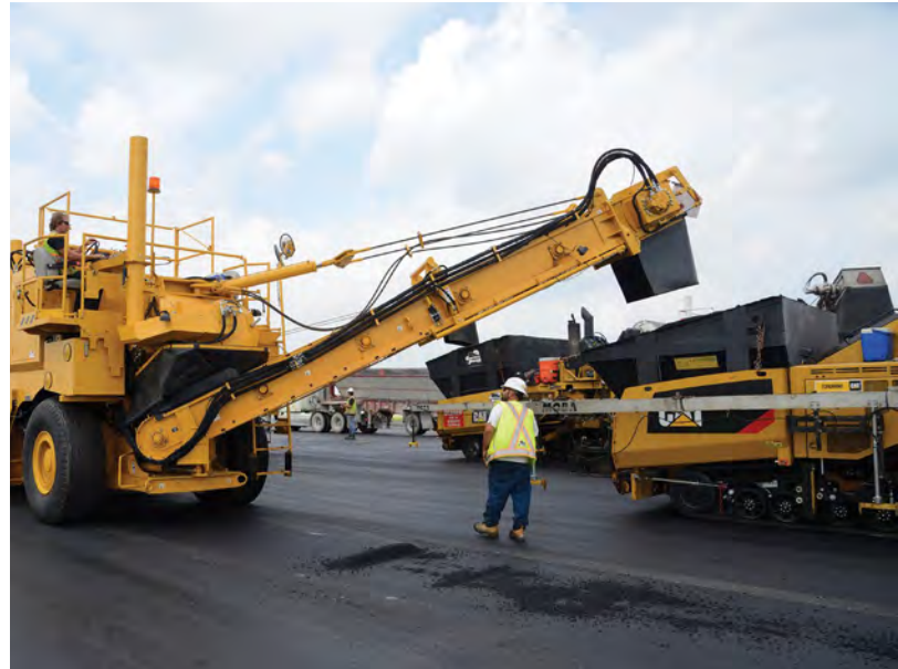
Crews need to avoid spills that can occur in front of material transfer vehicles.
