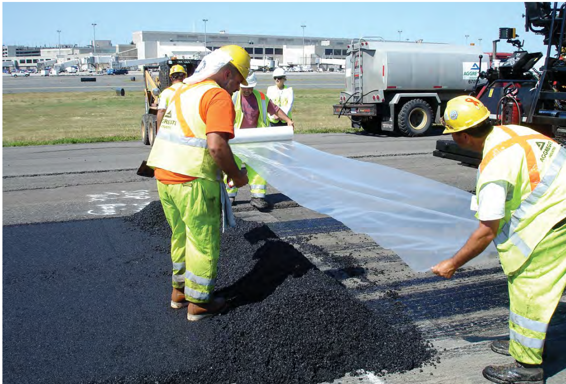
The end of a pass is prepared, so creating a butt joint is easy when paving resumes.
