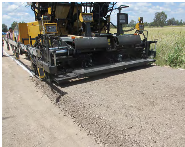
2.5 m (8') combination screed laying down aggregate base 3.5 m (11.5') wide and 30 cm (12") deep.
