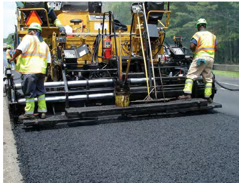
Stone-matrix asphalt is a stiff mix that is difficult to rake and shovel.
