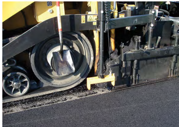
Sonic sensors use sound pulses to measure the profile of the grade over which the bituminous layer is being placed.
