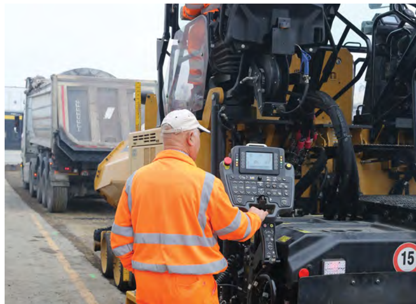
The paver continues to pave at normal speed as the empty truck pulls away.
