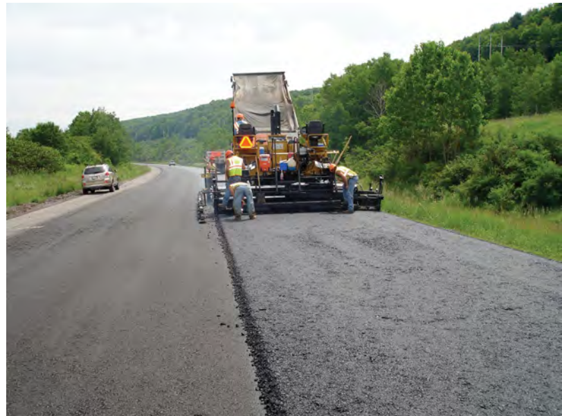
End-of-load segregation shows up at regular intervals as patches or V-shapes in the asphalt layer.
