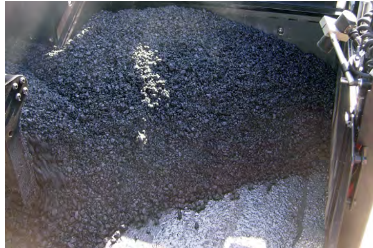
The screed operators' first responsibility is to make sure there is enough material in front of the extenders.
