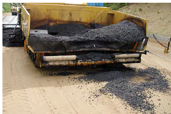
Improper truck alignment leads to hopper spills.
