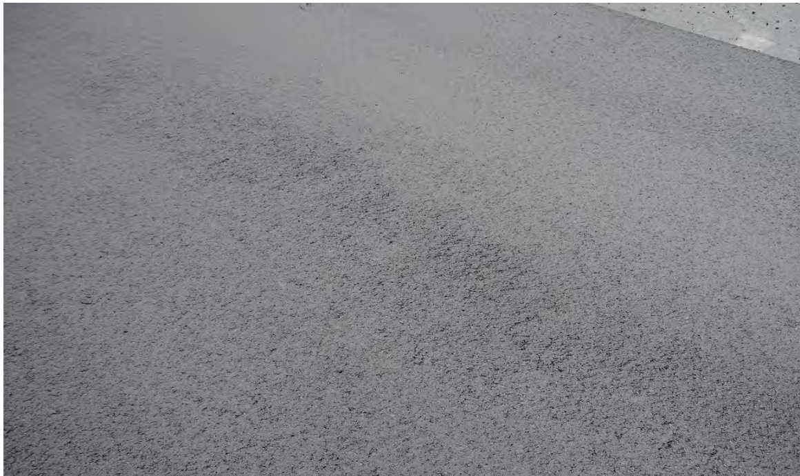
Drag mark caused by paving over compacted spill.
