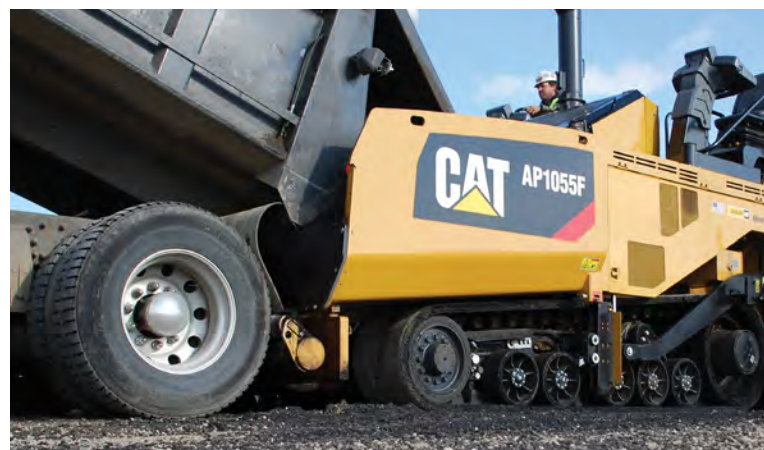
Two push rollers contact the rear tires of the haul unit as the paver pushes the haul unit.
