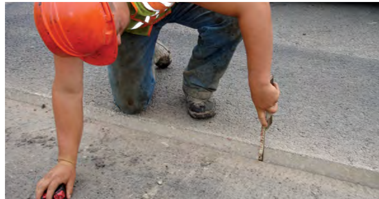
Measure the height of the butt joint to help select the correct starter board thickness.
