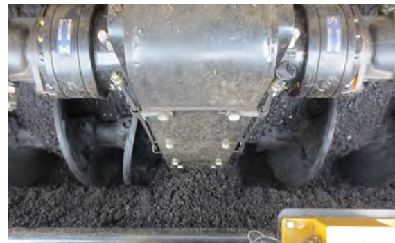
The head of material under and in front of the center chain case can be stagnant.
