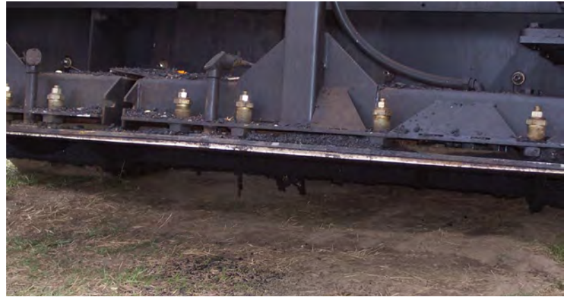
A wavy screed plate exerts uneven pressure and creates texture stripes.
