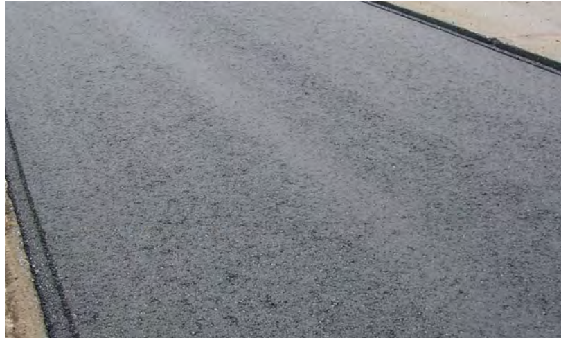
Running with the augers too low can cause two areas of open texture directly behind the auger shafts.
