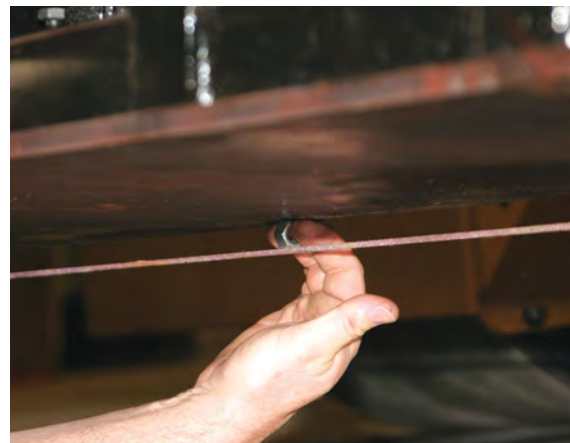
Installing 3 mm (0.125") lead crown in the main screed plate helps reduce centerline striping.
