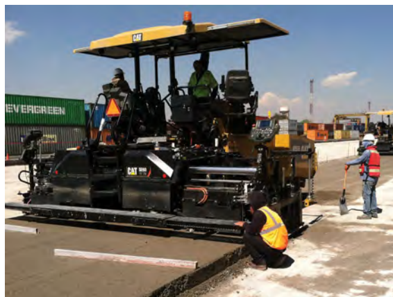
Thick layers of roller-compacted concrete are normally laid down with combination screeds.
