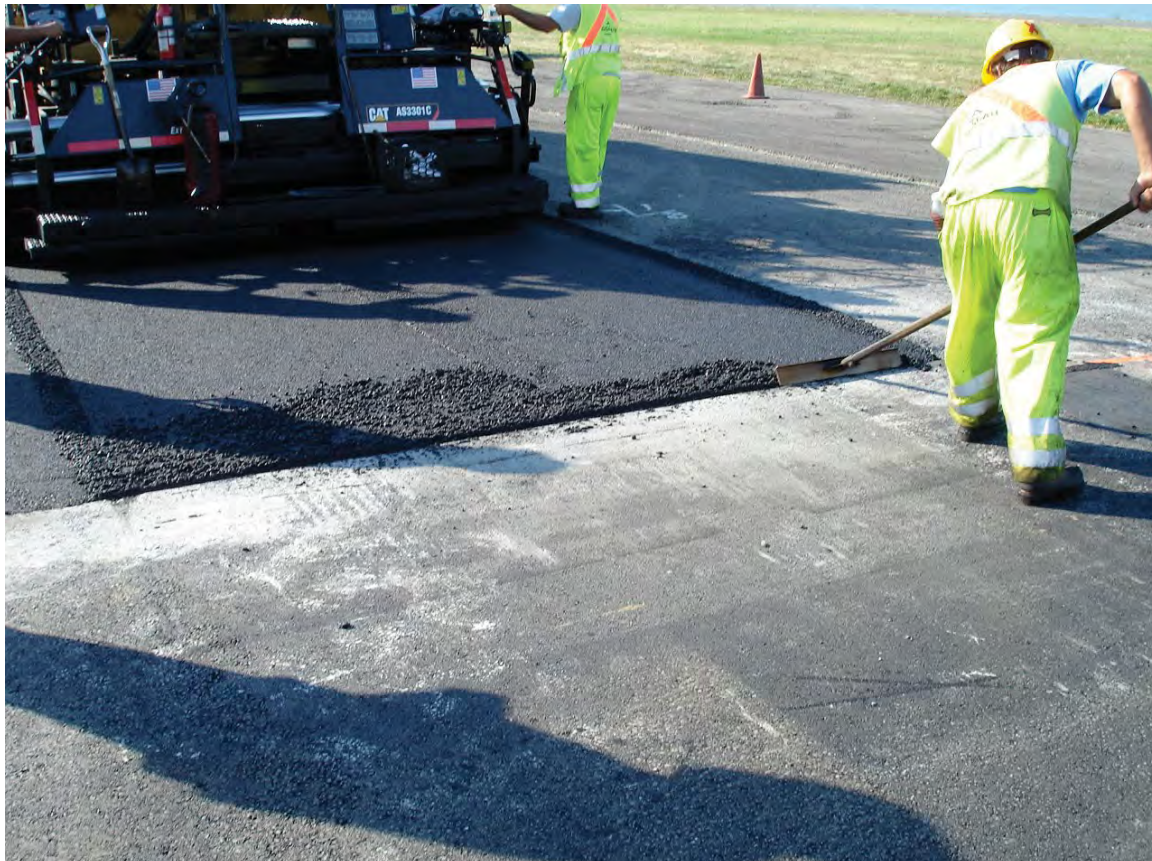
A properly built transverse butt joint requires minimal handwork prior to compaction.
