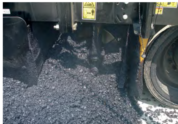
Mechanical feeder sensors contact the material as it flows out of the auger chamber.
