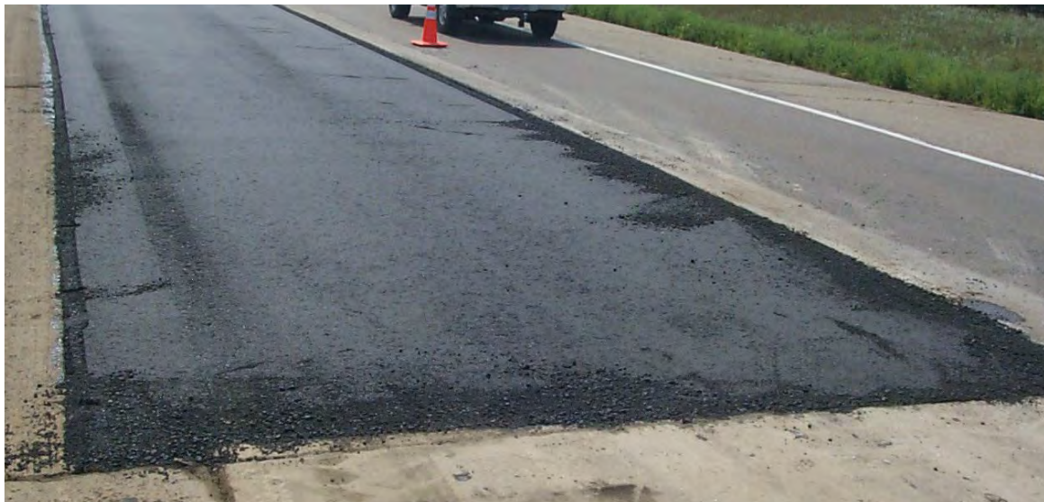
A screed that is not properly heated or that has cold sections will create drag marks and texture stripes.
