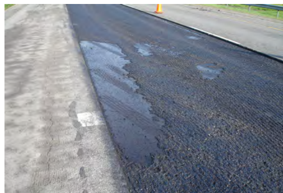
If the milled surface has areas of delamination, the milling depth may need adjustment.
