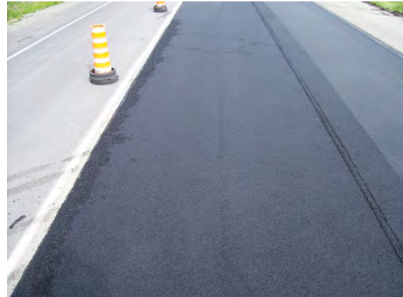
A centerline stripe can be caused by insufficient lead crown.
