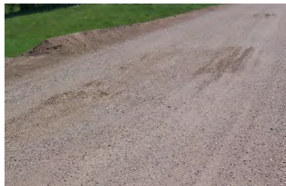
Substandard base, like this weak area, must be identified and repaired prior to paving.
