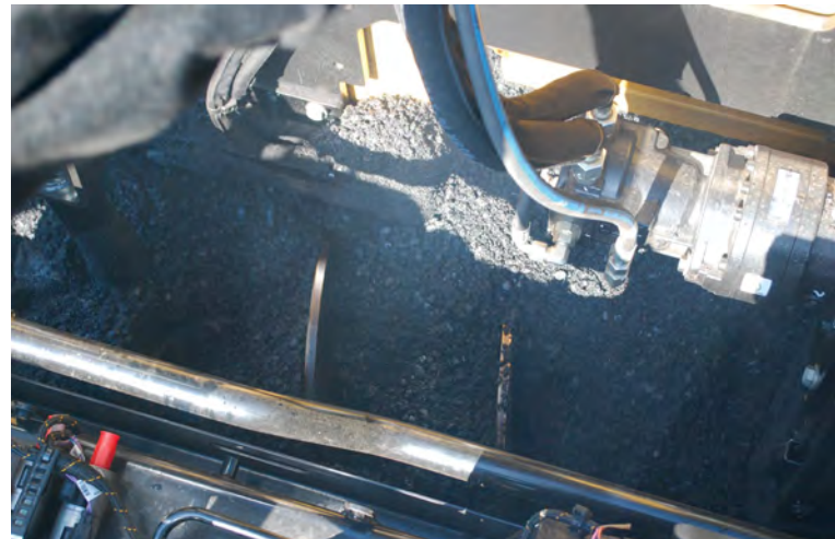
The paver operator checks the head of material in the center of the auger chamber.
