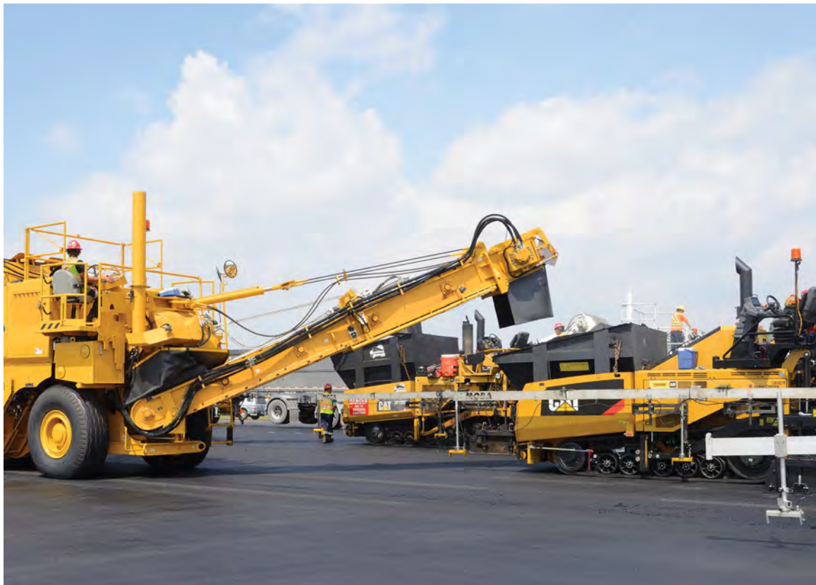
Run the first few loads directly through the transfer vehicle when the transfer vehicle is cold.
