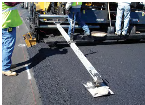
The rear section of the Fore 'N Aft Leveler rides on the new bituminous layer.
