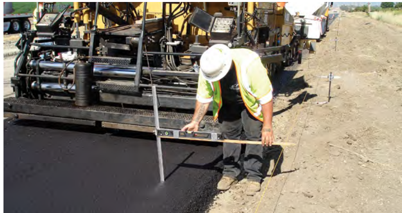
Controlling base layer elevation with an erected stringline on new highway construction.
