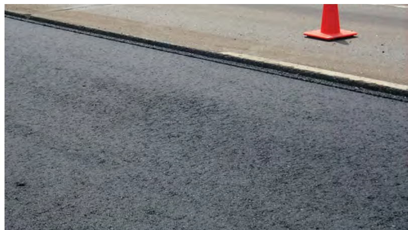
Temporary texture stripes caused by paving over high spot in milled surface.
