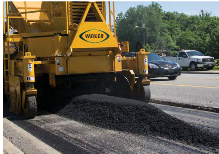
The end of a windrow often consists of segregated aggregates.
