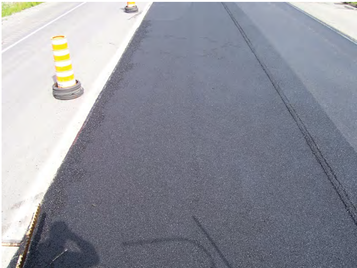
Centerline stripes can be related to feeder system operation.
