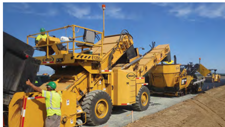
Use of a material transfer vehicle is frequently written into the specifications on highway projects in North America.
