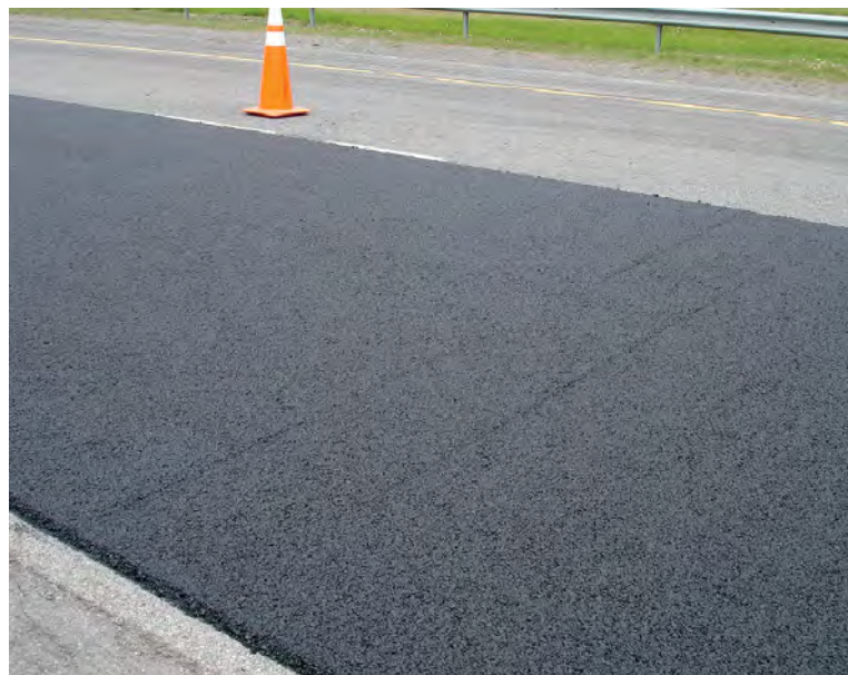
Stopping the paver during truck exchanges can cause a screed settlement mark.
