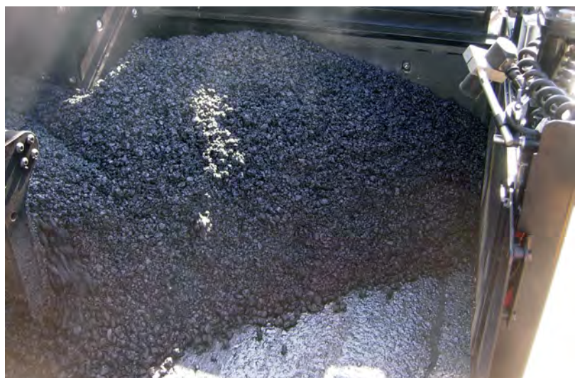
The screed operators are responsible for making sure enough material flows to the front of the extenders.
