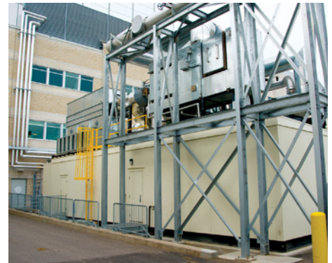
The CHP plant produces more than 16 million kWh of power and around 50 billion BTUs of heat per year.
