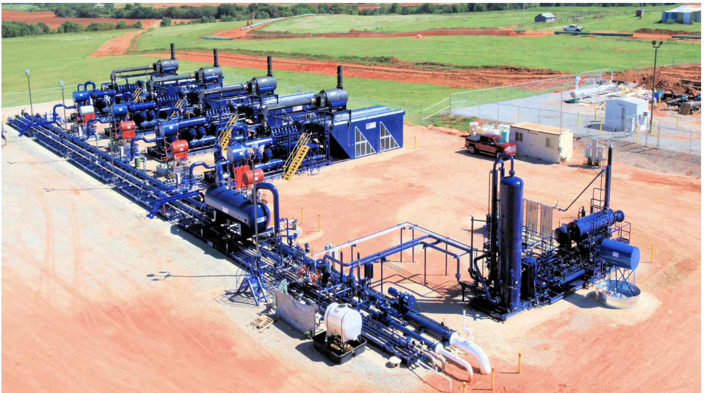
Compressor Station - USA Compression Partners, LP Powered by G3608 A4 engines
