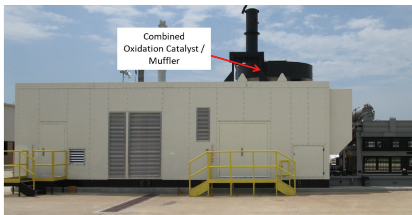
Figure 1: Oxidation catalyst integrated with muffler to control CO on a 2 MW gas generator set
