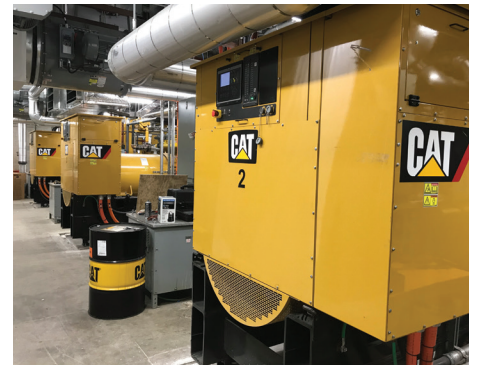
Last summer, Brock began replacing eight old Cat® G3516A workhorse engines with four Cat 3516H engines, which produce 2 MW of electricity each.
