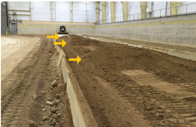
Operators started on a sand strip with three piles of sand to spread, simulating a truck dump application.
