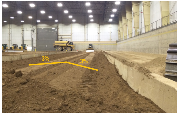
Slope Assist helped make quick work of building a road with a 3 percent crown.
