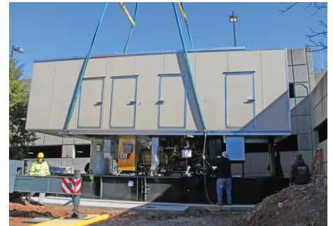
The Cat® C27 diesel generator set equipped with dual-fuel technology is surrounded by a soundattenuated enclosure to help reduce noise inside the city hall building and the surrounding residential neighborhood.
