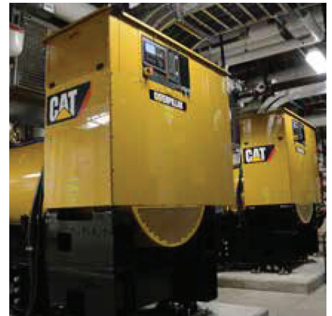
G3516H gas generator sets
