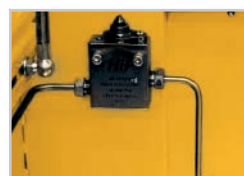
The flood and safety valve.
