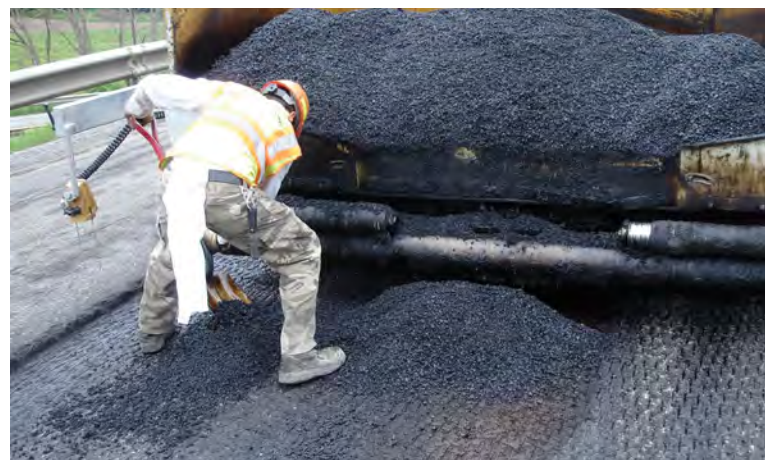
Spills on the grade in front of the paver are a big mistake and should be corrected.
