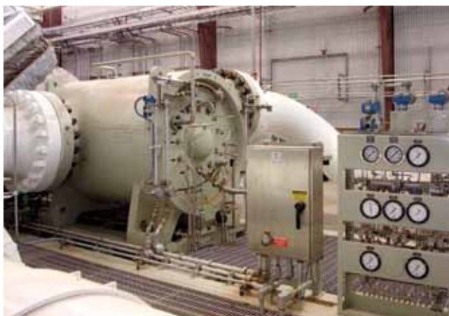
C65 Gas Compressor
