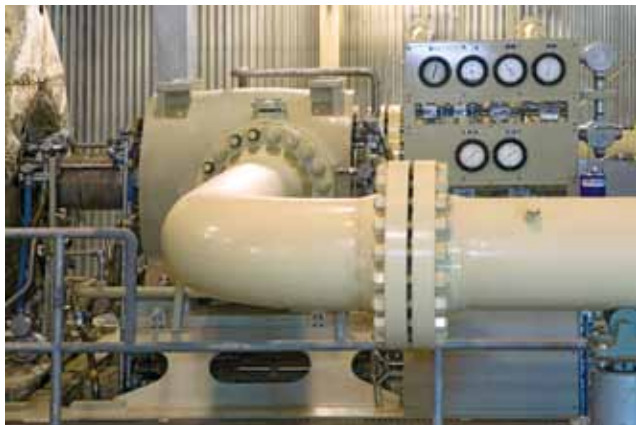
C33 Gas Compressor
