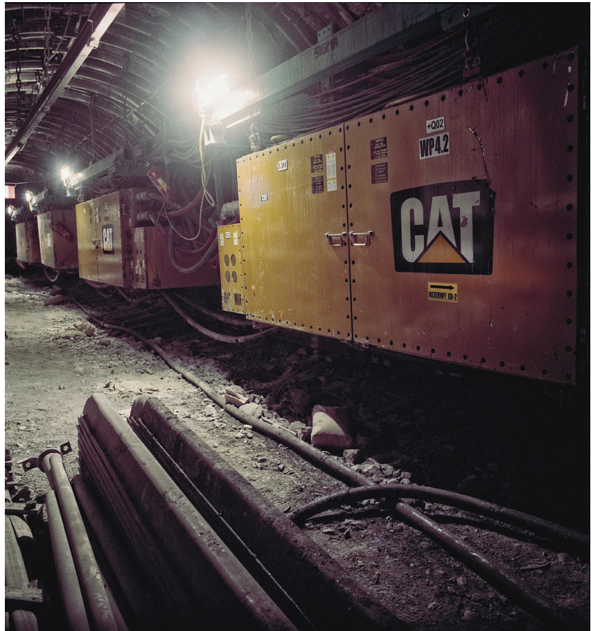
Cat VFD system at Bogdanka.
