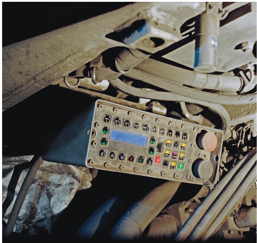
PMC-R roof support control underground.
