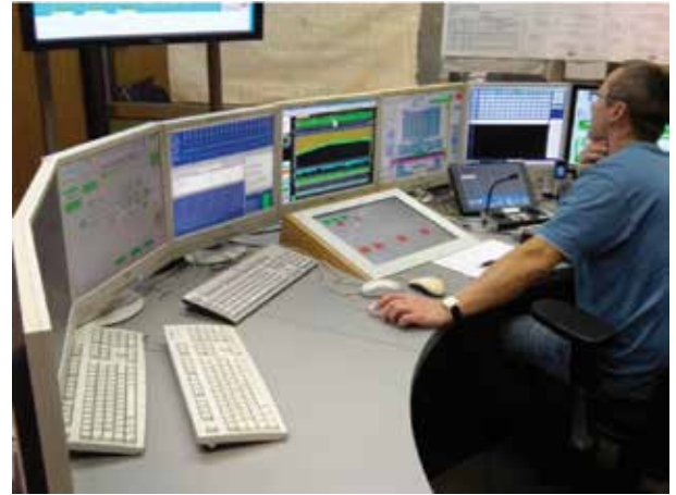
FIGURE 3. Surface control center at a German mine
