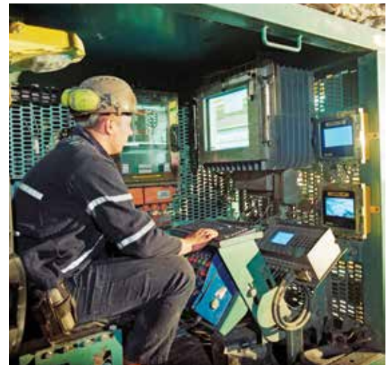
Underground longwall control cabin with face visualization
