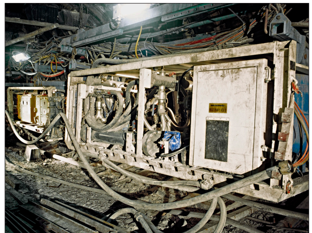
Separate Cooling Station
