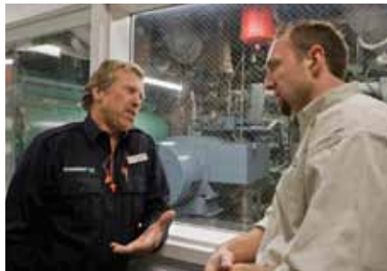
Snowbird staff follows a strict maintenance schedule to help ensure generator longevity.
