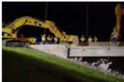
The rebuilding of this Dallas-Fort Worth highway is representative of needed infrastructure improvements in the developed world.
