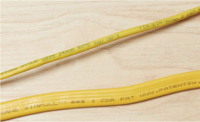
Picture of the field wiring to unit (Picture should clearly show wire gauge)
