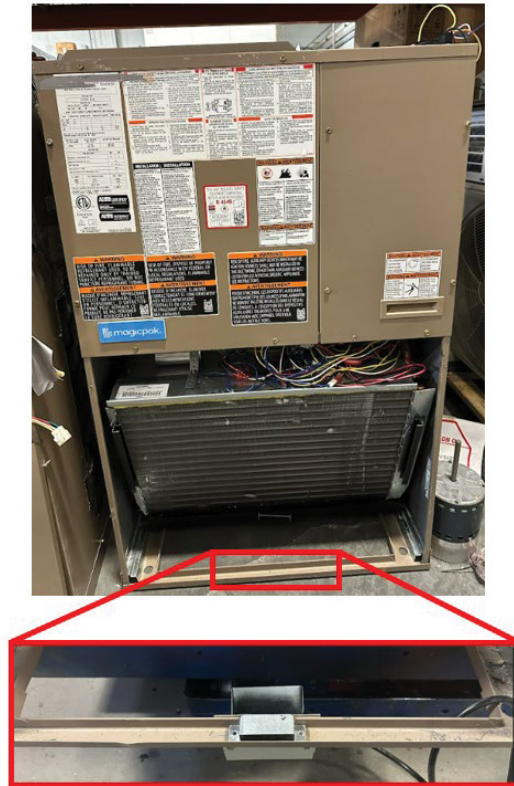
RDS Sensor Installation
