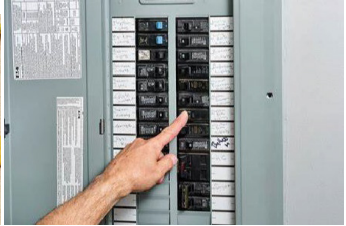
Picture of overcurrent protection (Picture should clearly show breaker size)
