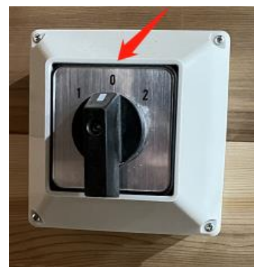
Power turned OFF
