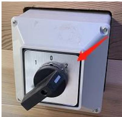
Power to Infrared heaters
