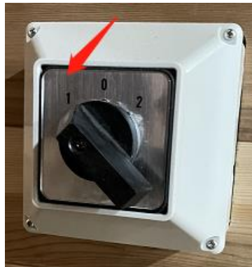
Power to stove heater
