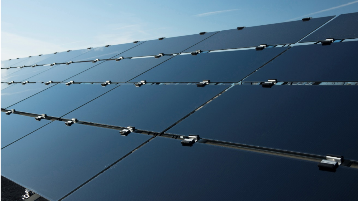
Figure 3. Typical thin film PV array on racking system and clips.
