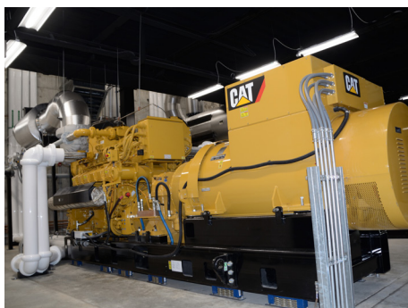
The new plant cuts the resort's carbon footprint in half, saving 62,000 dekatherms of natural gas each year.
