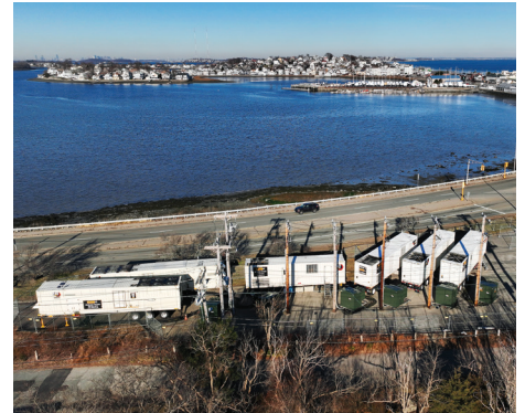
Following a day-long power outage in 2020, the Town of Hull acted to protect itself, renting five Cat® XQ2000 power modules that produce a combined 10 MW of power.
