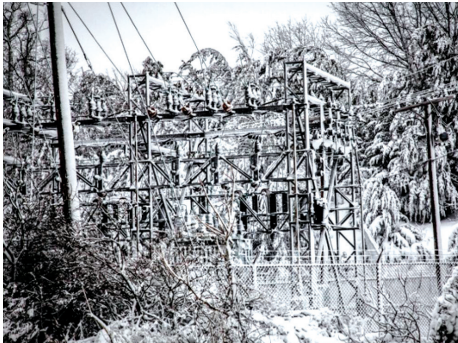
In recent years, a combination of strong storms and aging transmission lines has led to 13 power failures.
