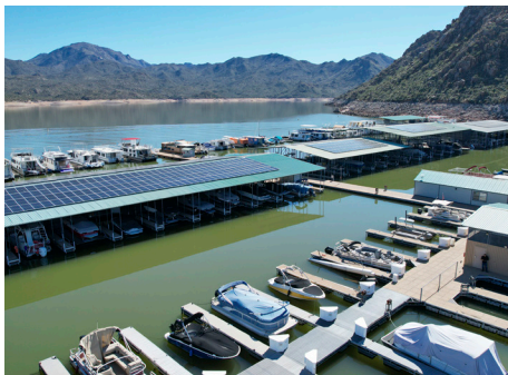
Bartlett Lake's microgrid consists of a 400 kW solar array with 895 solar panels mounted on the roof of the boat slips that provide power to the marina.
