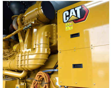
A Cat® C175 genset at Colby's municipal power plant. Colby ran their first C175 for 38 consecutive hours during Winter Storm Uri in 2021.
