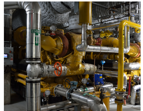
A portion of a combined heat and power system at an HHS hospital, which is powered by Cat® G3516H natural gas generator sets. CHP systems from Caterpillar can provide total energy efficiencies up to 90 percent.
