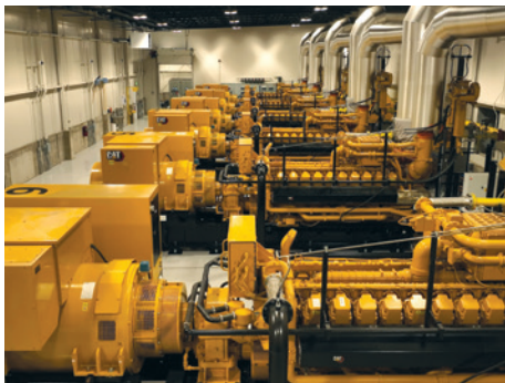
Cat® dealer Wheeler Power Systems supplied the generator sets and assisted with design and construction of Solomon Generating Station in St. George, Utah.
