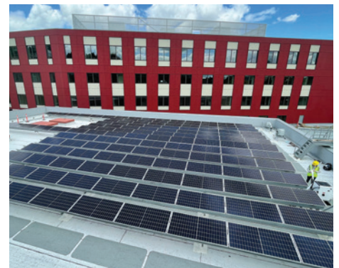
Lincoln High School's hybrid microgrid includes a 278 kW Cat solar array.
