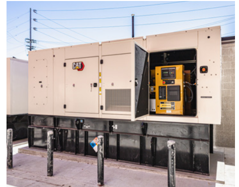
In the event of a grid outage, two Cat® diesel generator sets, a C9 and C13, are prepared to provide standby power to Portland's Lincoln High School.
