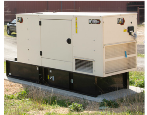
A new Cat D100 GC generator set provides standby power to a pump station in the event of an outage.
