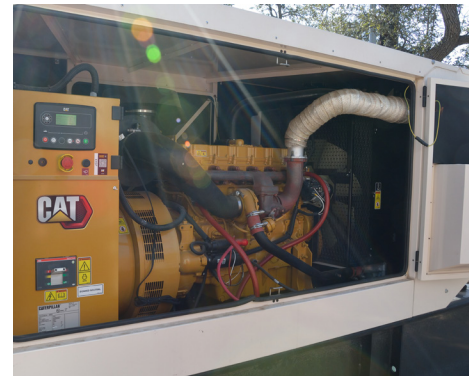
A new Cat D200 GC generator set is the newest addition to a fleet of four other Cat gensets that provide backup power to operations at Natural Bridge Caverns.
