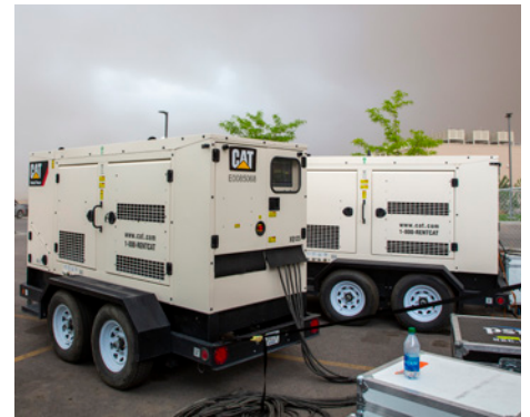
Cat mobile generators are connected to rented RVs that serve as artists’ green rooms at the Shoshone-Bannock Casino Hotel’s outdoor venue in Fort Hall, Idaho.
