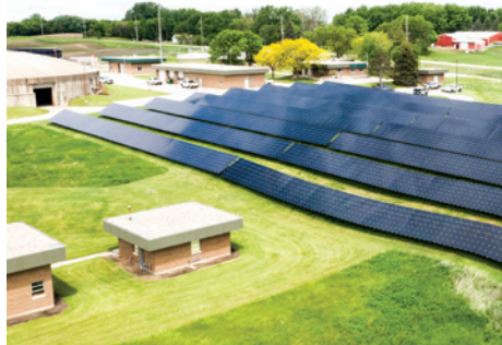
The solar array performs well in the heat and humidity of the Upper Midwest's sunny weather.
