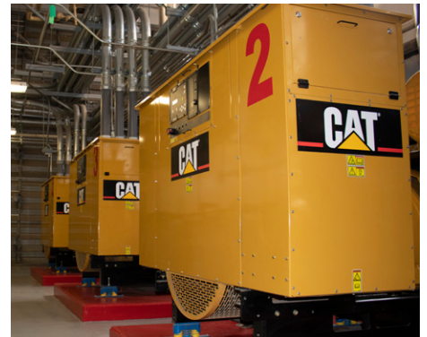
Three Cat C32 generator sets helped OSF St. Francis Medical Center in Peoria maintain power during an emergency outage in February 2022.
