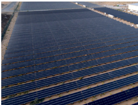
The system features nearly 23,000 Cat® PVT117 photovoltaic modules that generate up to 2.7 MW of solar power for the facility during daylight hours.
